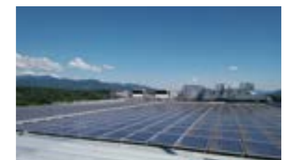
Solar power generation system at ULVAC COATING CORPORATION
