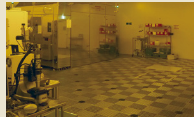
Super clean room of Federal Standard Class 1 In January 2014, “F7000S-VD02” a new ultra high-speed electron beam drawing device was installed here.
