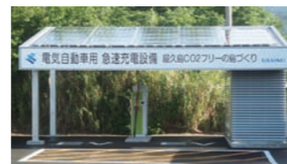
Electric vehicle quick-charging station with a power storage function
