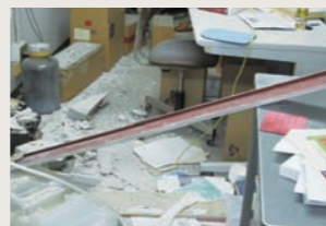
A collapsed column in Building B at the Tsukuba Institute for Super Materials
