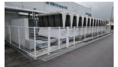
Cold/hot water heat source equipment
