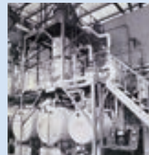
High-vacuum distillation equipment for plasticizers
