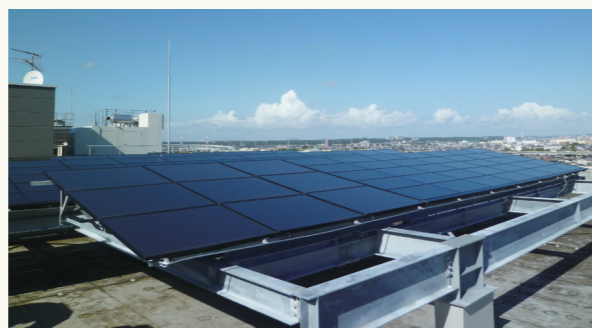
Solar power generation facilities within the Head Office and Plant in Chigasaki, Kanagawa
